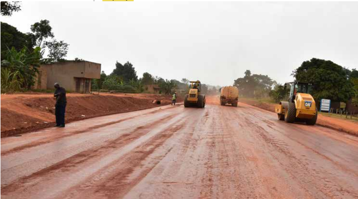
Ongoing earth works on Mubende Kakumiro Kagadi Road project by Armpass Technical Services, a local contractor and member of UNABCEC.
