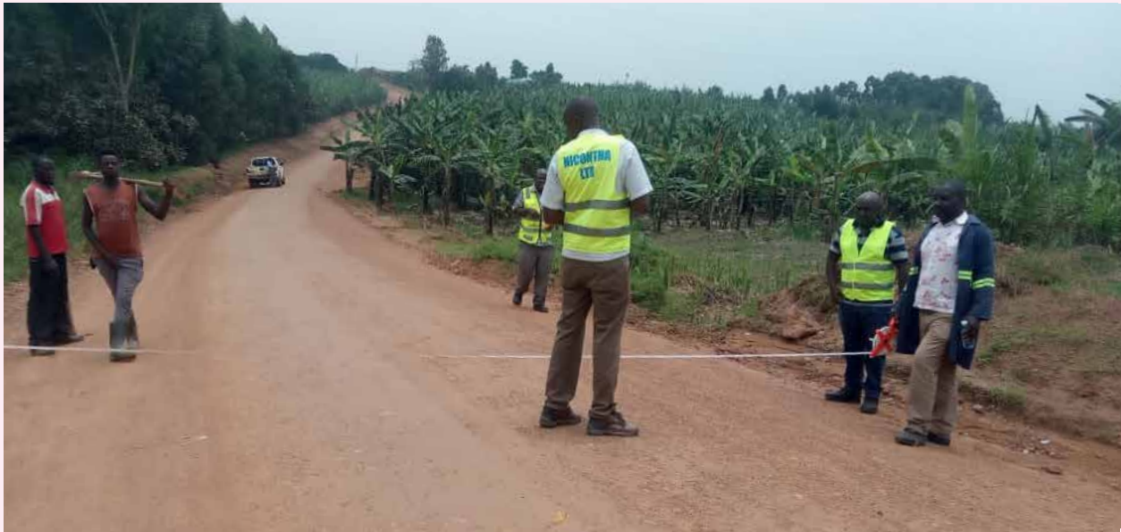
NICONTRA LTD and UNRA team carry out joint measurements for field density tests, gravel thickness and width of the Kahunga - Nyakyera - Rukoni road project
