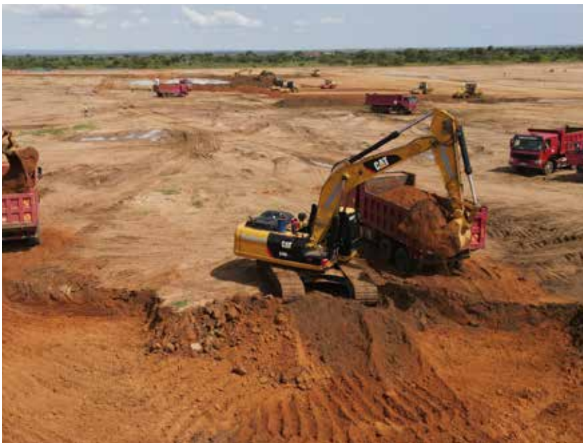
Ongoing works by Civtec Africa Ltd, one of the UNABCEC Members executing works in the oil and gas sector.
