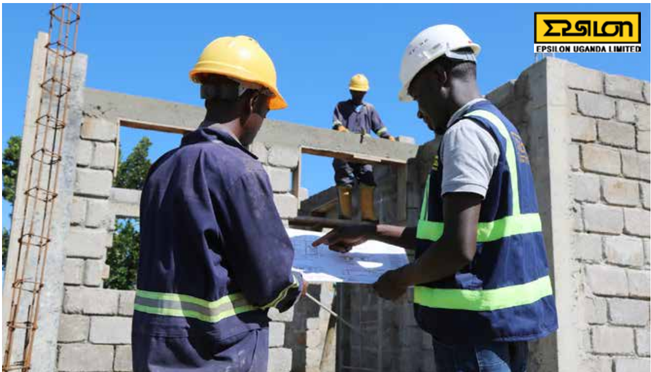
Gideon (Right) interpreting a construction drawing to a Site Foreman during the Construction of EACOP Replacement Houses in Lwengo District.
