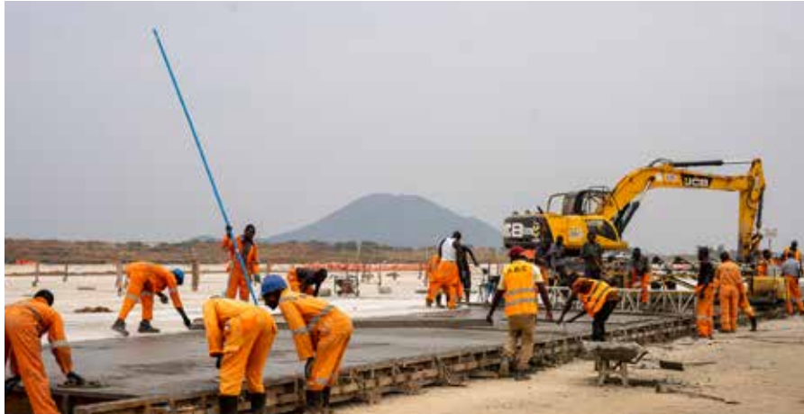
Ongoing construction works at Kabale International Airport by SBI International Holdings Uganda
