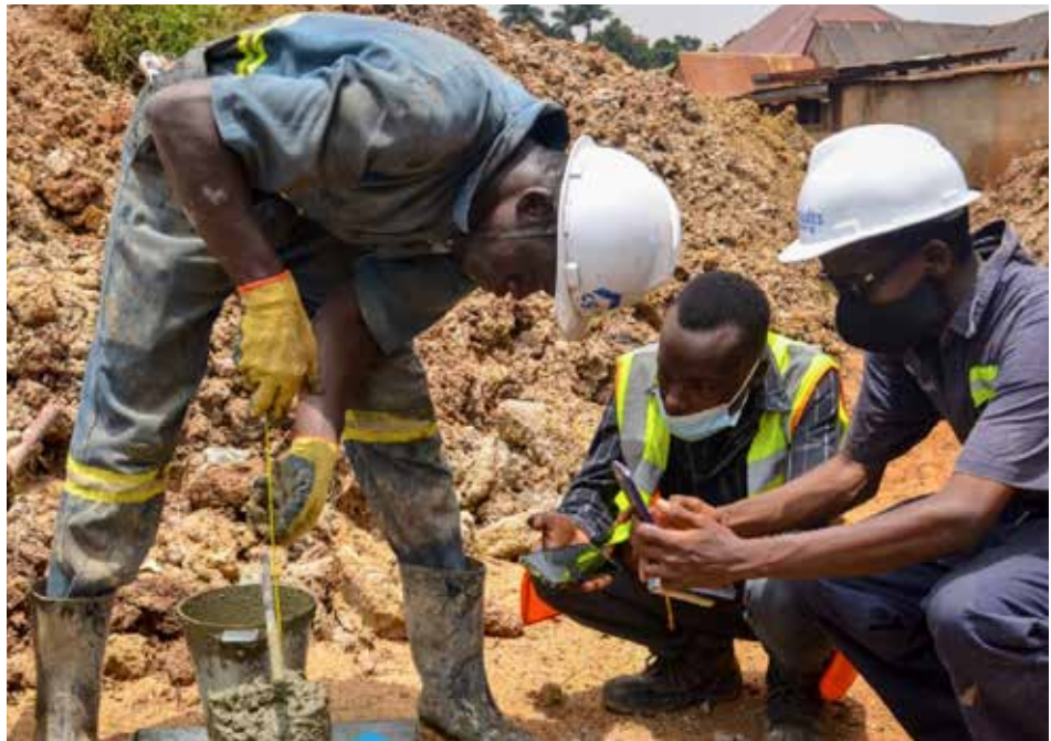
Checking for concrete slump at a drainage improvement works project in Kawempe, Kampala city by CG Engineering Consults staff and a member of the consultant's team.
