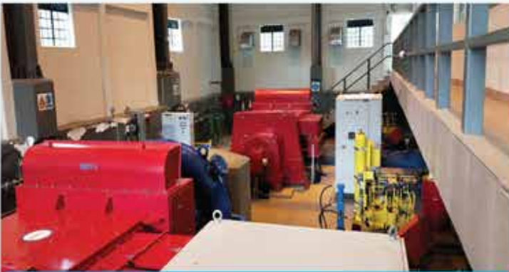
Completed installation of Turbines in Power House Waki, Hoima
