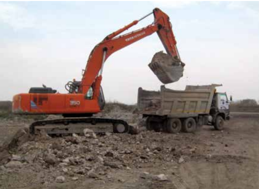
Teclon Ex350 & LPK2523 at work for Kasese Nail & Wood Industry Ltd
